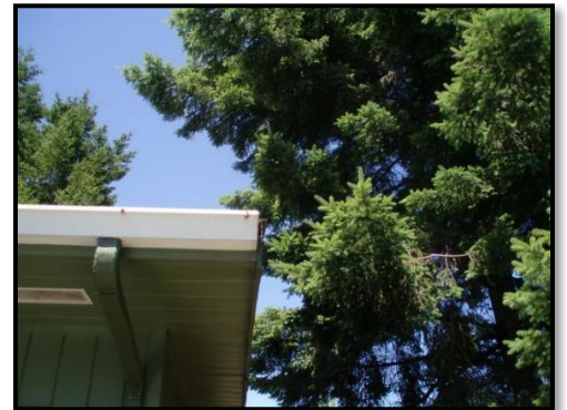
Branches against the roof.
